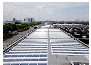
Fujisawa Plant's solar power panels
