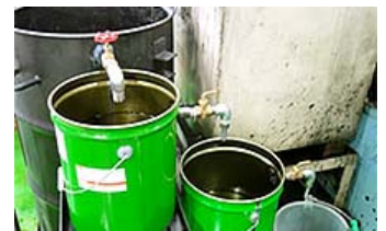
Waste oil separation device
