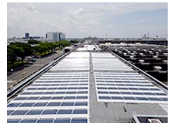
Fujisawa Plant's solar power panels
