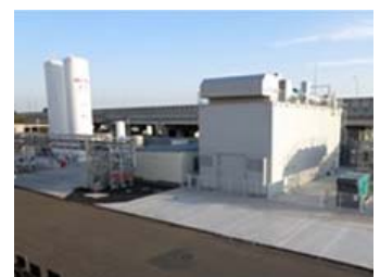
Tochigi Plant Co-generation System
