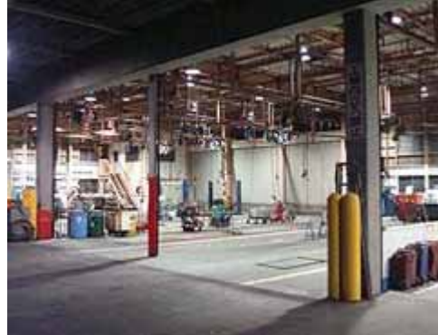
Replacing lamps in a service workshop (Mercury lamps -> ceramic metal halide lights + Adaptive diode lighting)
