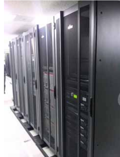
New energy saving data servers
