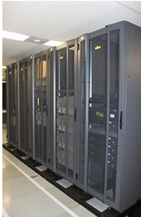
New energy-saving server
