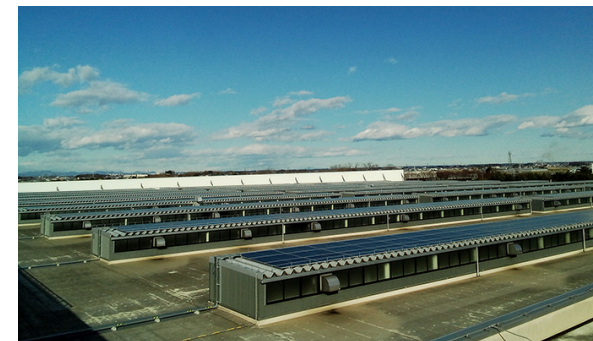
Solar Power Generation Facility at the Tochigi Plant
