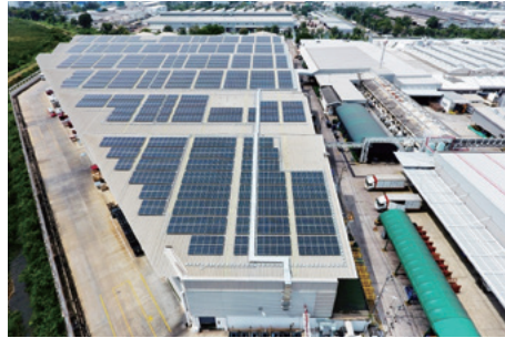
Isuzu Engine Manufacturing Co., (Thailand) Ltd. (IEMT) solar panels
